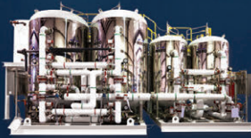
Carbon Filters & Softeners
